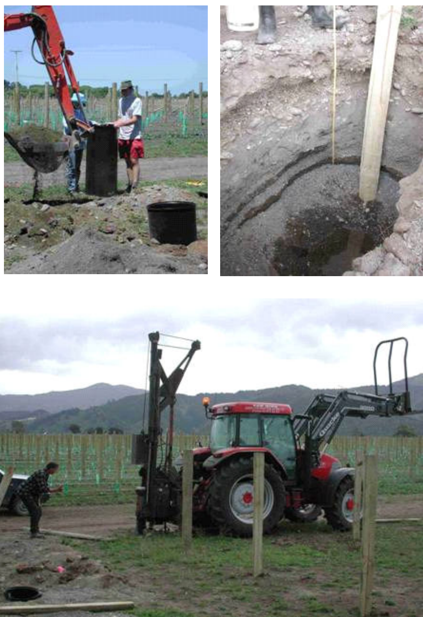
Figure 1. Installation of the posts and lysimeters at Delegats, Rarangi. The photos (top left) show the installation of the lysimeters, the nature of the shallow groundwater (top right), and the driving in of the other posts (bottom).
